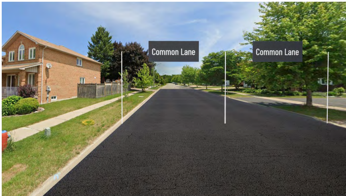
Figure 3-2: Existing Conditions on Briggs Avenue between Bayview Avenue and Edinburgh Drive – (Looking east)
